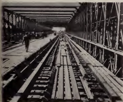
Elevated rail tracks ready for removal, the trolley tracks still in place.
